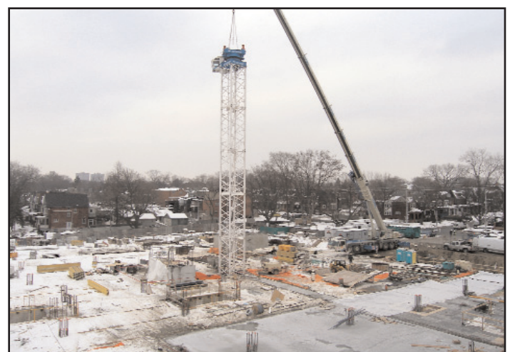
Top picture shows a view of the redevelopment site and the top of the parking garage.
