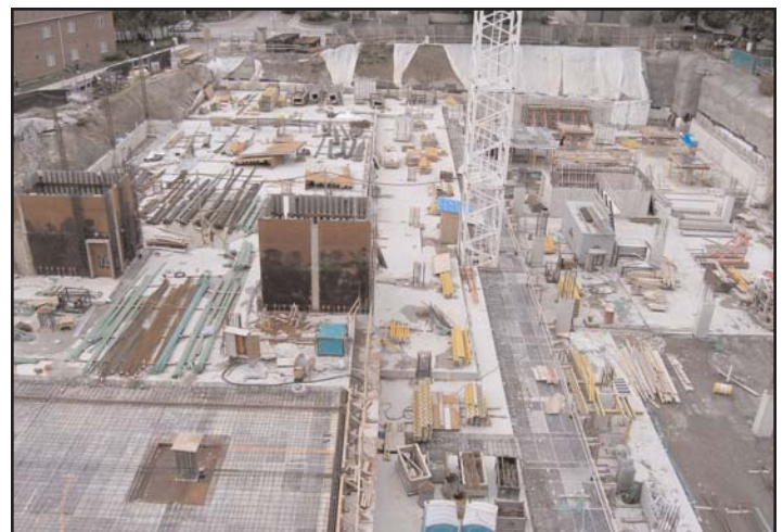
Top & bottom pictures show the progress made to date on the underground parking garage.
