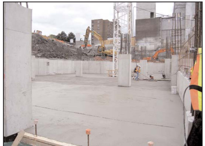
Top picture: View of parking garage construction and site. Bottom picture: Concrete slab for underground parking garage
