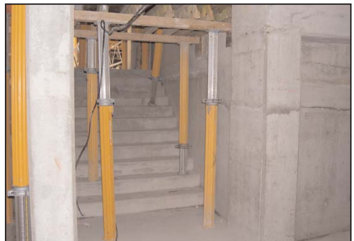
Top picture: Construction of underground parking garage Bottom picture: Bottom P3 of underground parking garage
