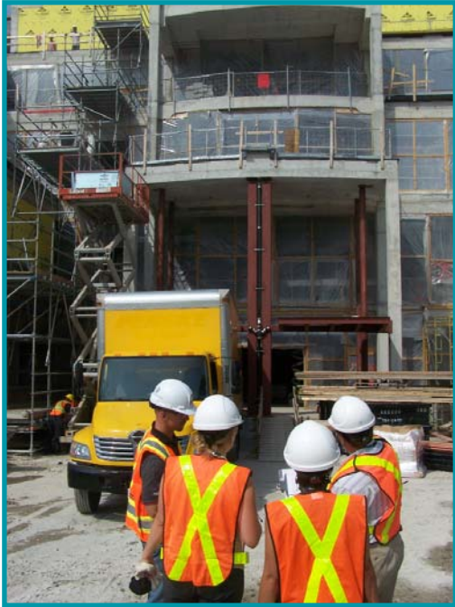
Beginning the tour out front of the new Our Lady of Mercy wing entrance.
