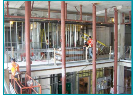
The large poles in the centre will hold the stained glass from the original building.
