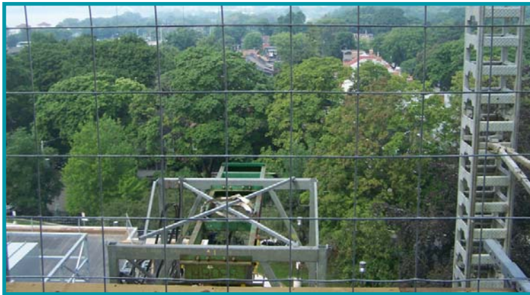
The fifth floor mechanical room looking out over our catchment area.
