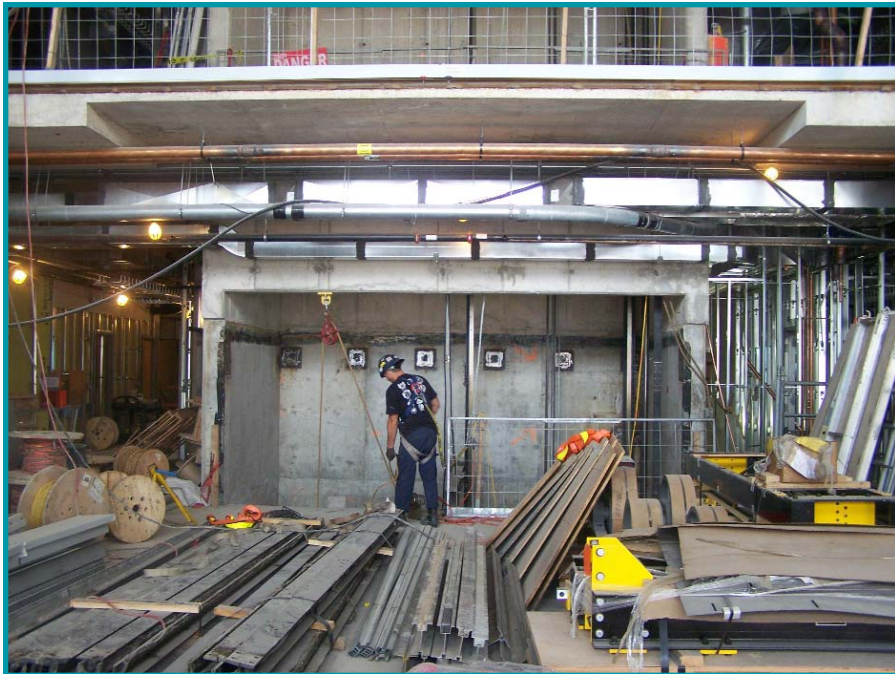
The first floor foyer and main elevator shaft of the new wing.
